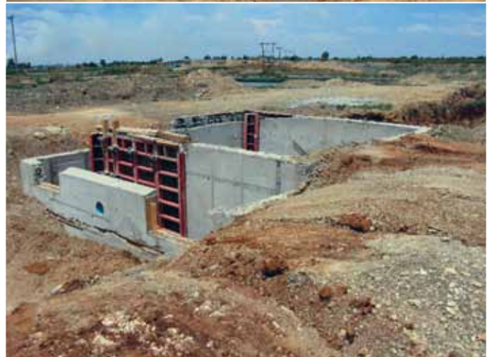
Pictured above construction work in progress at the Jan Kempdorp Treatment Works.
