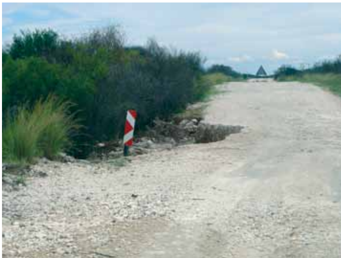
The destruction to gravel road surfaces in the DMA. The road pictured above is located between Blikfontein and Boetsap farms.
